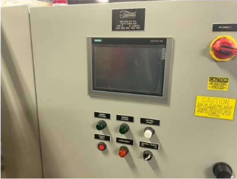
Control Panel Exterior
