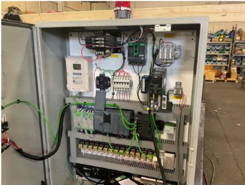
Control Panel Interior
